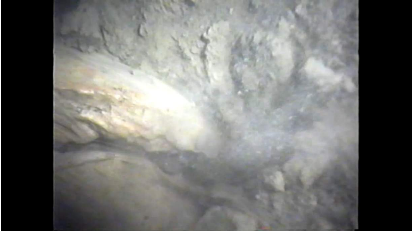
2007 Leaking Pipe Joints
